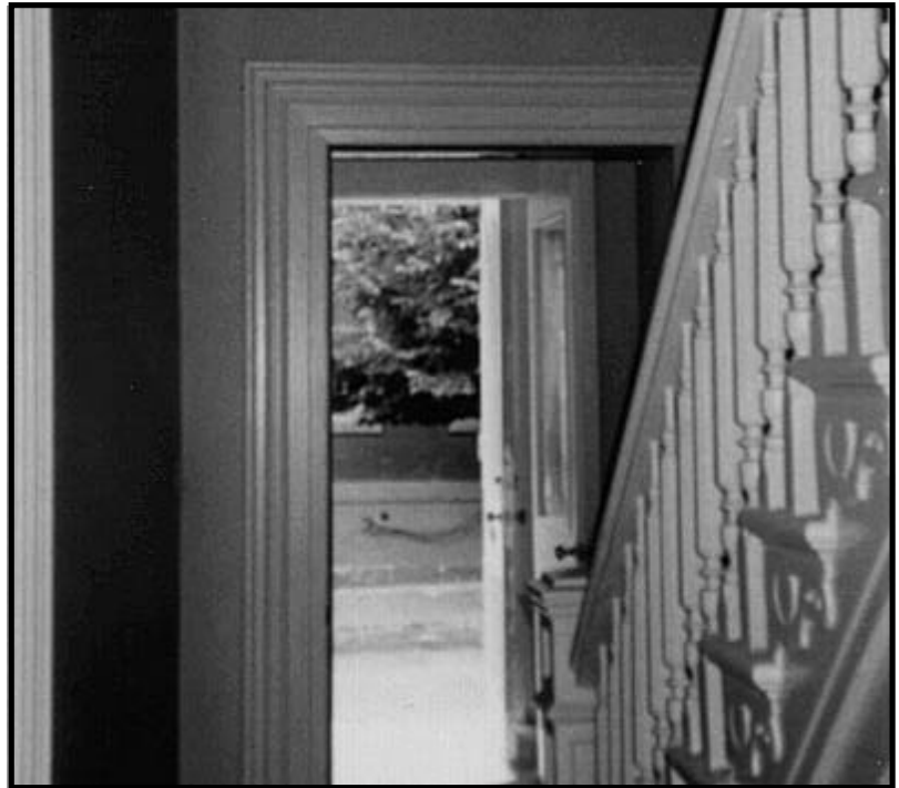
Figure 18.3 Historic Property Where the Interior Woodwork and Staircase Were Wet Sanded and Recoated With Three Layers of Encapsulant To Preserve the Carved Profiles.
